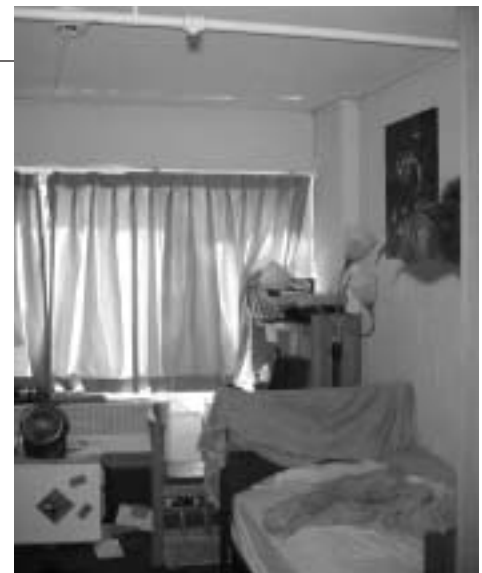
This Northwestern University dorm room was recently retrofitted with a fire sprinkler system. All NU dorms will be protected with fire sprinklers as part of a five-year plan.
