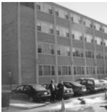
Sprinkler fitters test the capacity of the new fire pump in front of Elder Hall. Three hundred students live in dorm.
