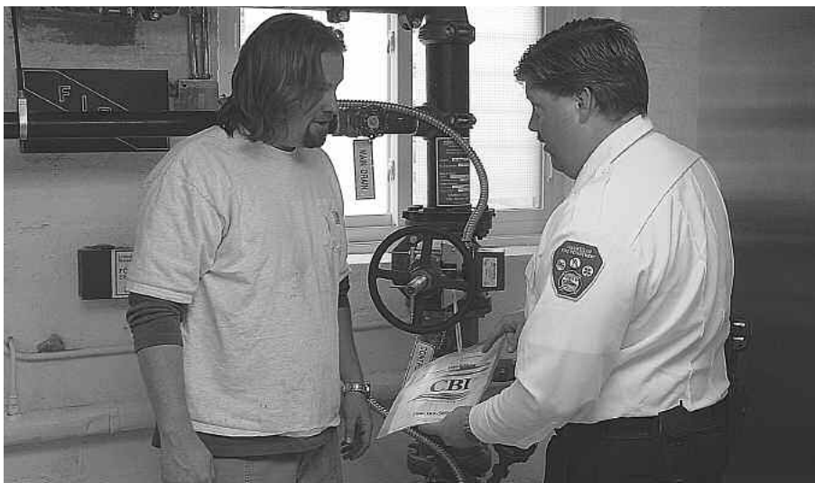
Waukegan Fire Marshal Steve Lenzi and Community Social Services Administrator Dennis Mudd check out the fire sprinkler riser.
