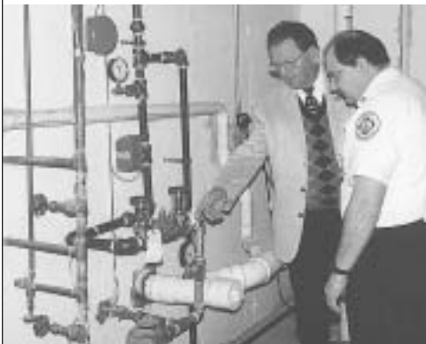
Chief Don Mobley and Chief Dave Danley check out the riser in the basement of the Glenkirk home right after the system was activated.
